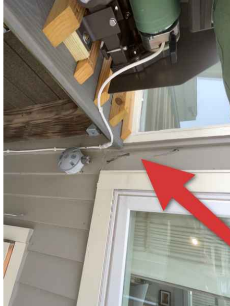
Minor paint chipping
