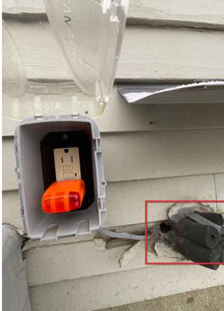
Hole in exterior siding.
